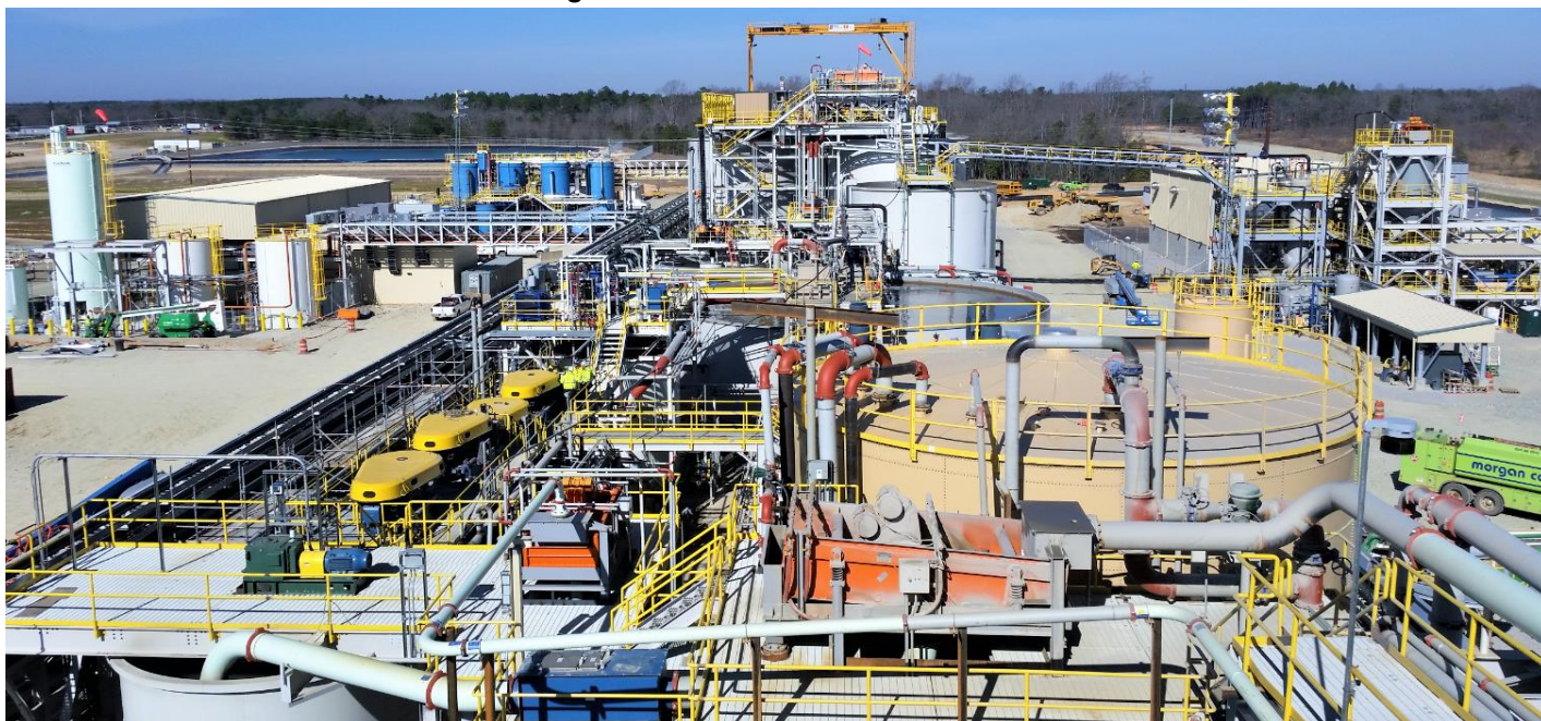
Figure 3 – Process Plant Overview
